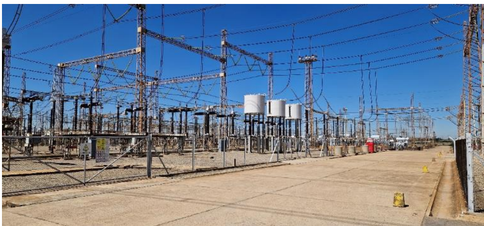
Figure 9-67: Street and fences substation Apollo 400/275 kV
