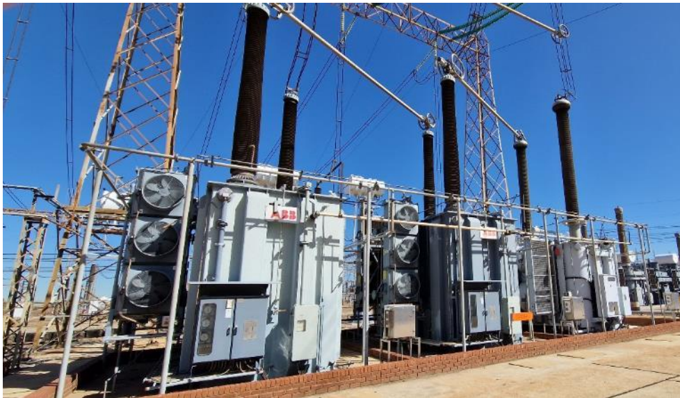
Figure 9-41 Transformers Apollo Converter Station 530 kV DC/275 kV AC
