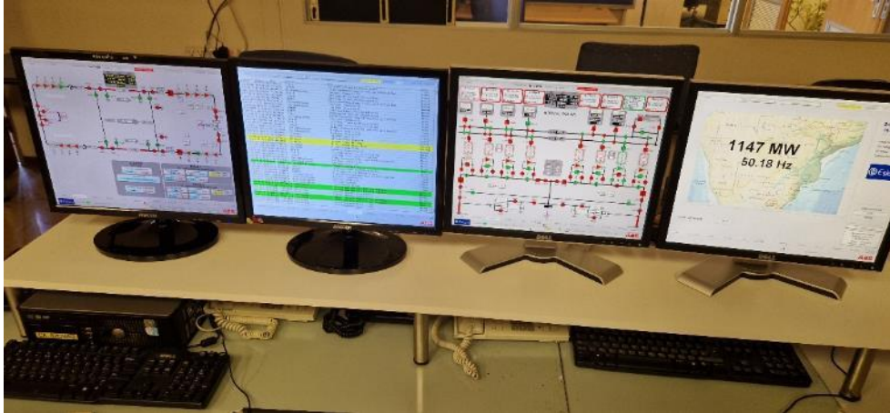
Figure 9-44: Control desk Apollo Converter Station 530 kV DC/275 kV AC
