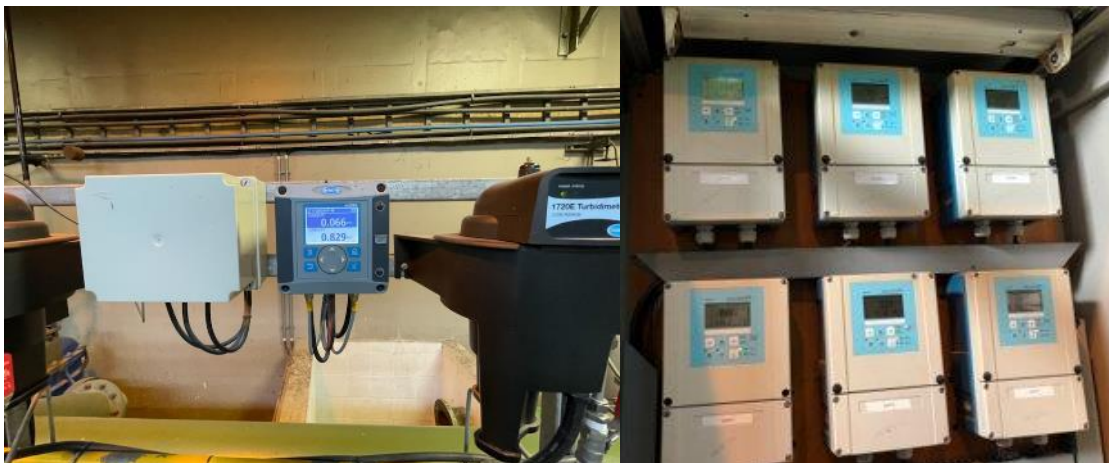
Figure 114: Measurement at Kriel's water treatment plant
