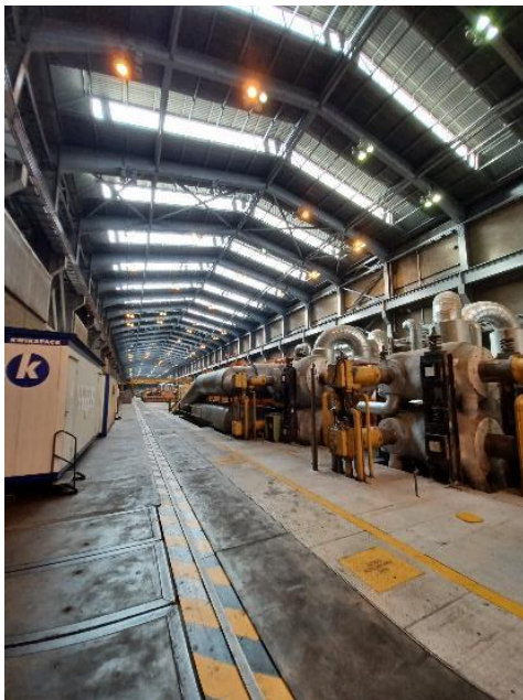
Figure 136: Turbine hall at Lethabo power plant
