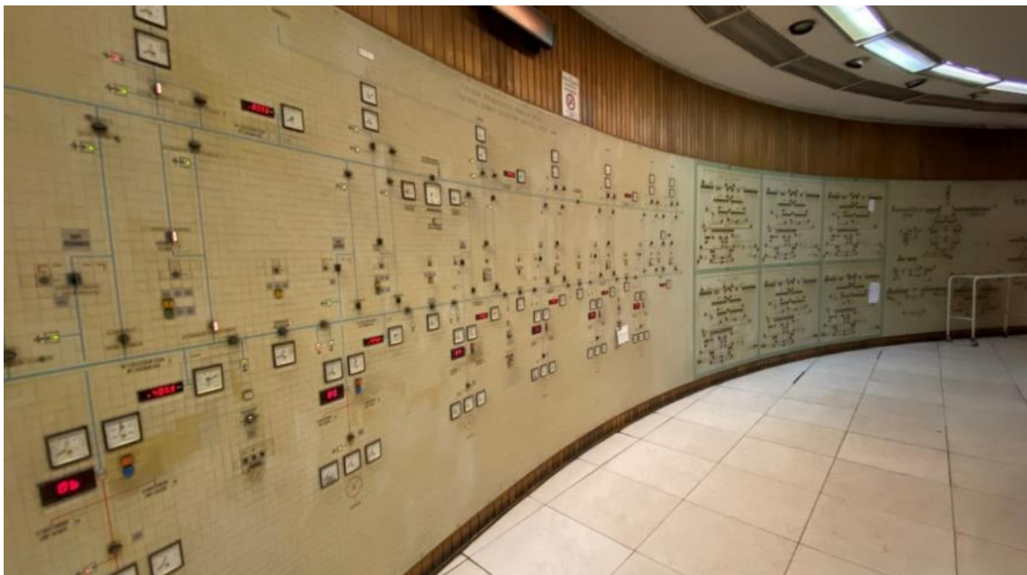
Figure 193: Mosaic panel HMI board at Tutuka power plant
