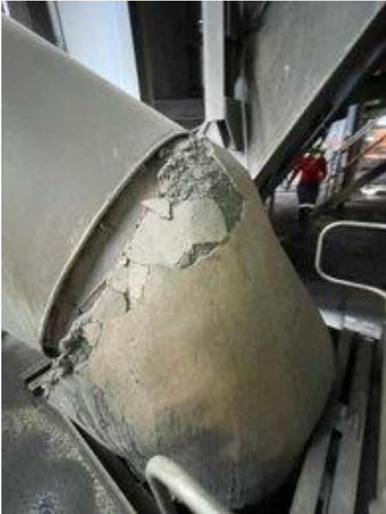
Figure 107: Example of cracked plaster insulation at a pipe in Kriel's boiler house
