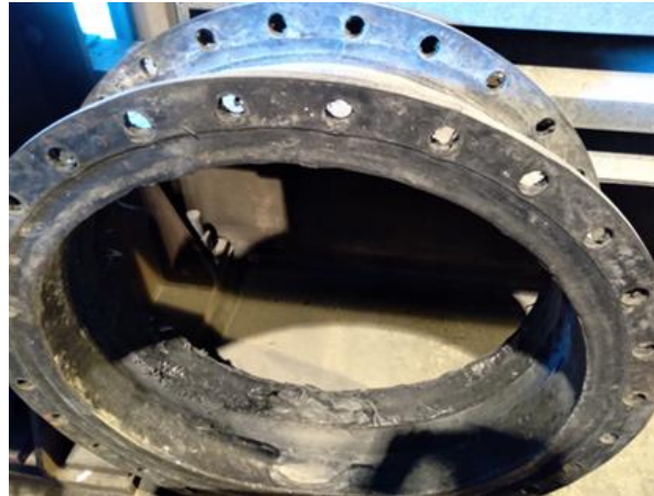
Figure 119: Damaged rubber liner at Kusile
