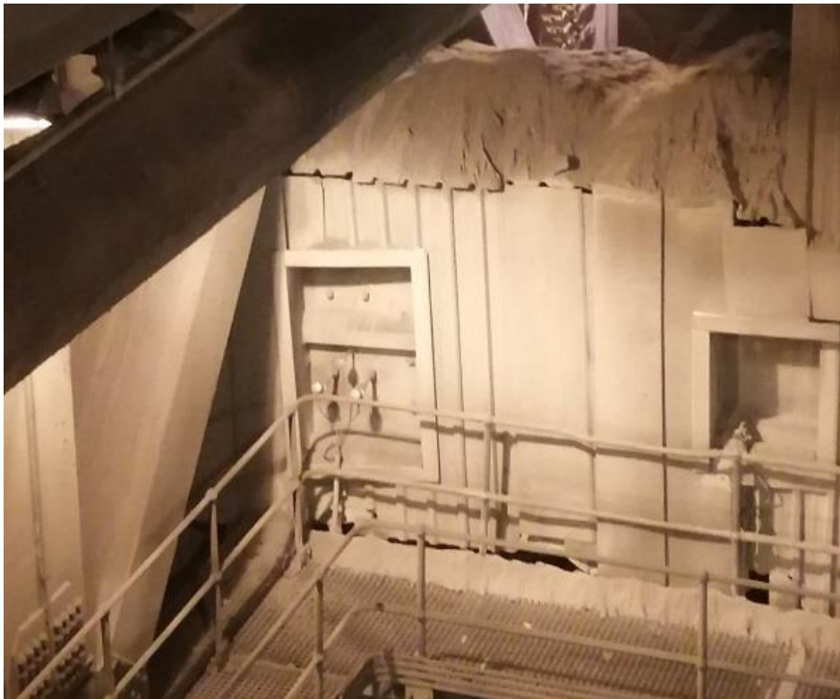
Figure 95: Kendal Unit 2 – PAH duct covered in ash and dust (April 2023)
