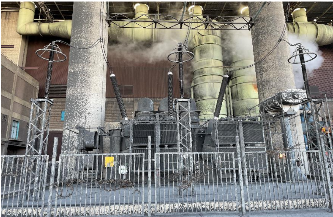
Figure 148: Soiled transformer at Majuba power plant Covered in grease and oil from the ACC fans
