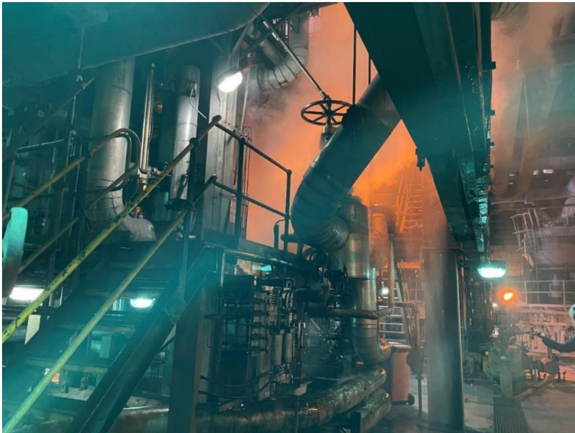
Figure 52: Steam leakages on the lower floors of the Camden machinery house
