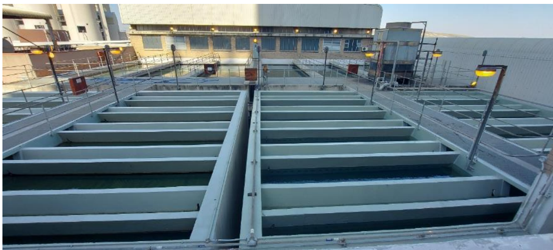
Figure 153: Sand filters at the water treatment plant at Majuba power plant
