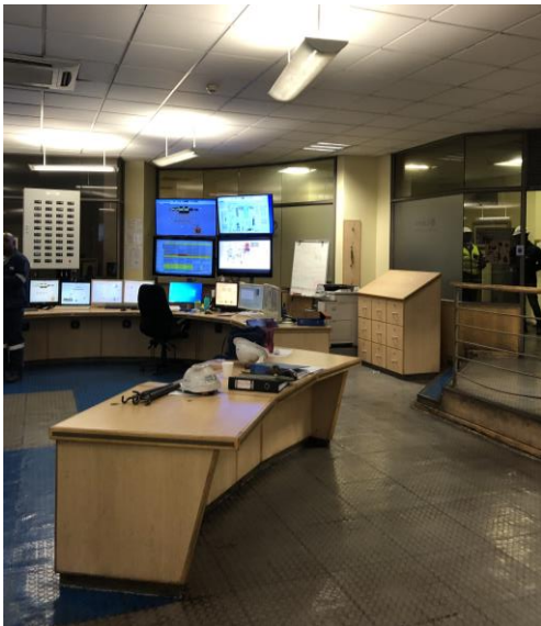
Figure 112: Control room at Kriel
