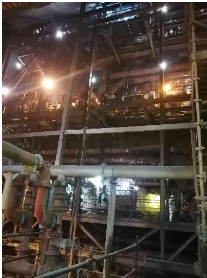
Figure 132: Lethabo's Unit 6 boiler house
