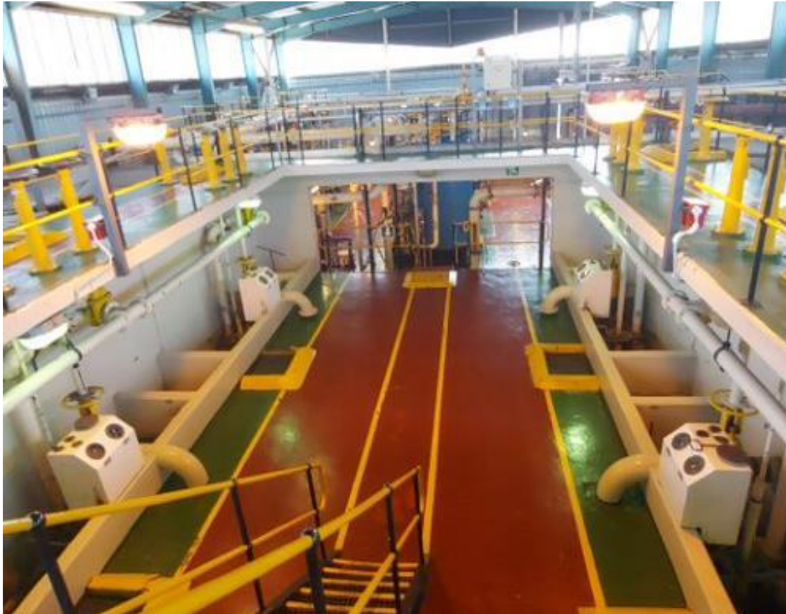
Figure 54: Water treatment plant at Camden power plant
