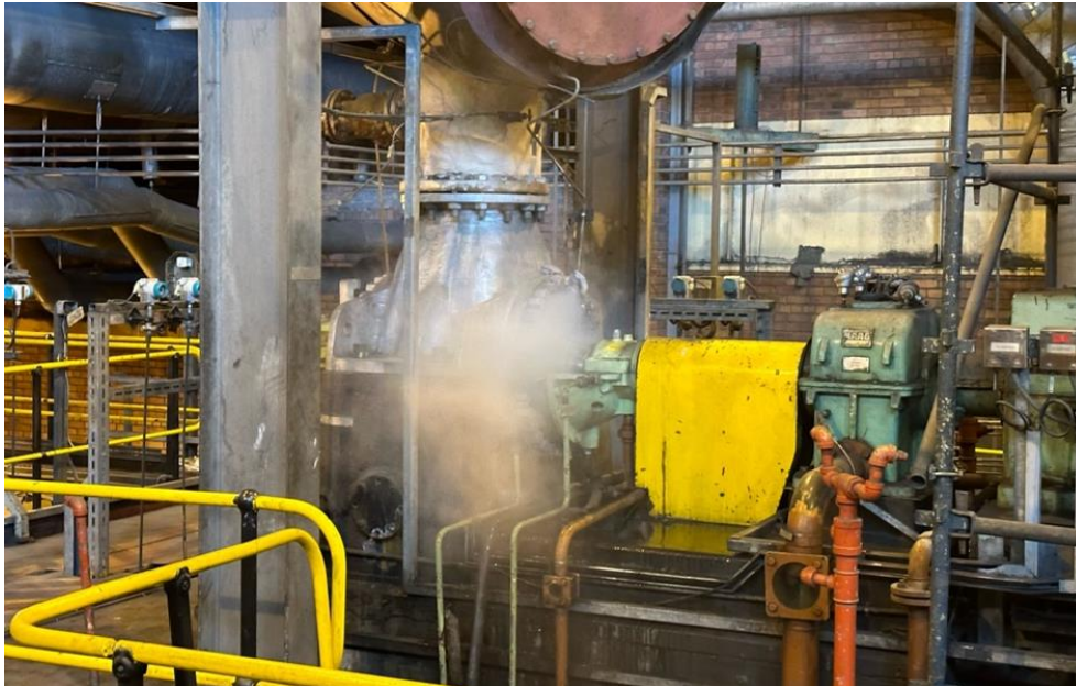
Figure 62: Leaking pump in Duvha's boiler house
