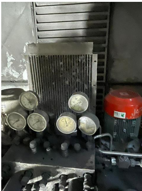
Figure 111: Oil station at Kriell's HP bypass
