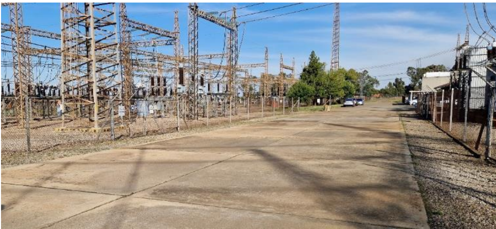
Figure 9-31: Street and fences substation Eiger
