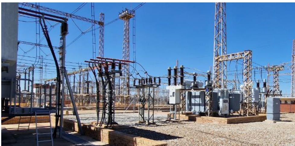
Figure 9-63: Part of auxiliary system substation Apollo 400/275 kV
