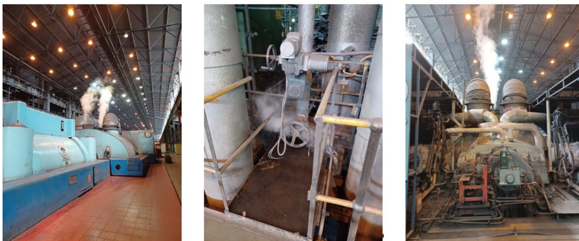
Figure 88: Turbine hall at Hendrina
