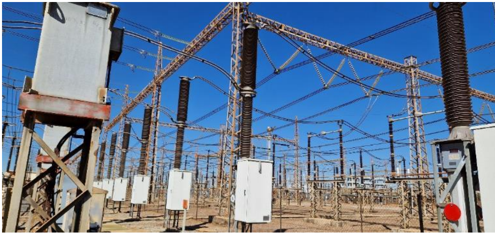
Figure 9-52: 275 kV switchgear Apollo Converter Station 530 kV DC/275 kV AC
