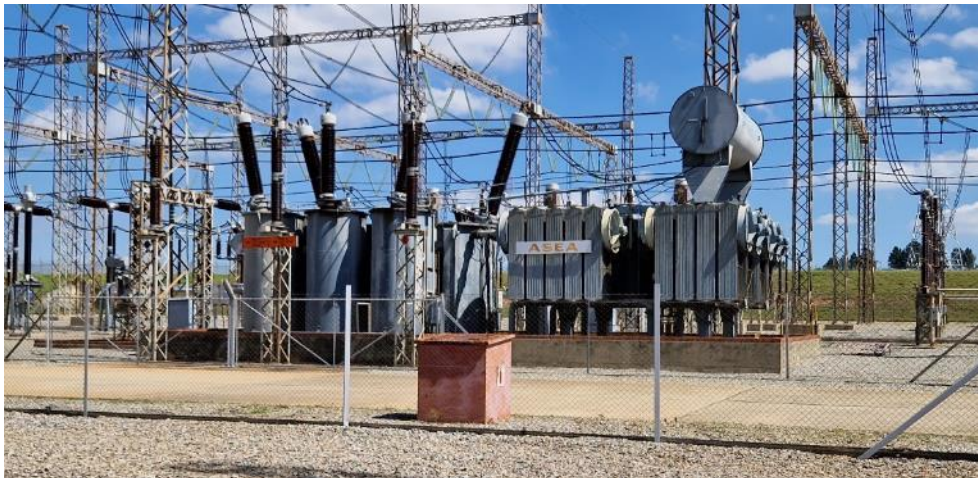
Figure 222: Power Transformer in substation Minerva
