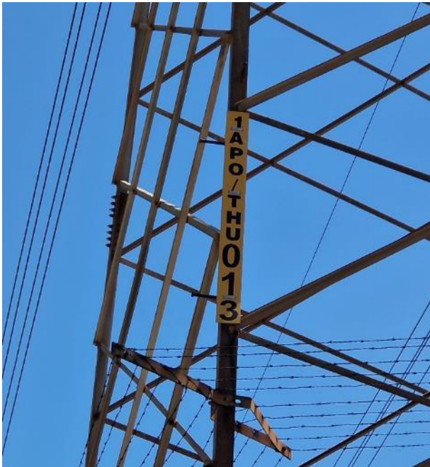
Figure 244: Marking of tower 1APO/THU013.
