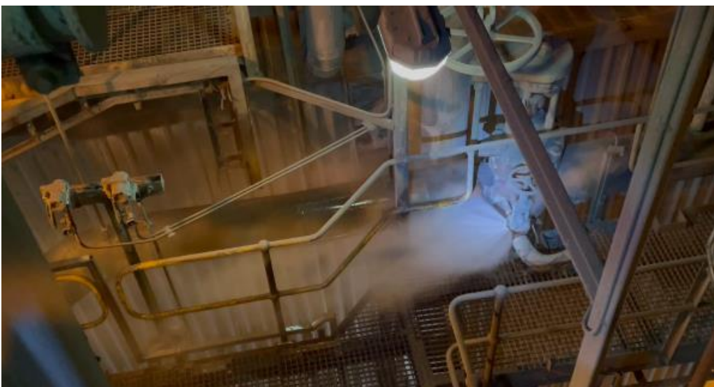
Figure 45: Valve leakages in Camden's boiler house
