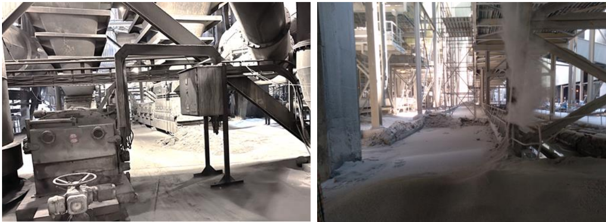
Figure 157: Poor housekeeping in Matimba's boiler house
