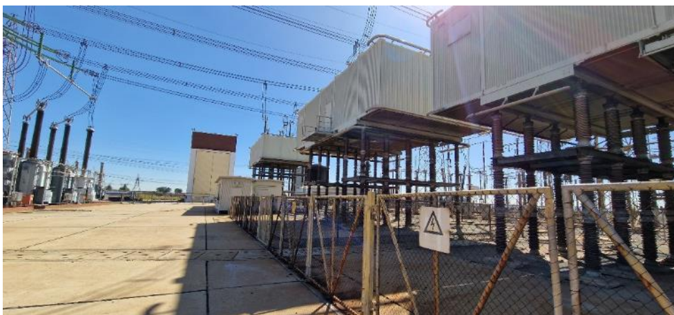
Figure 9-48: Street and fences Apollo Converter Station 530 kV DC/275 kV AC
