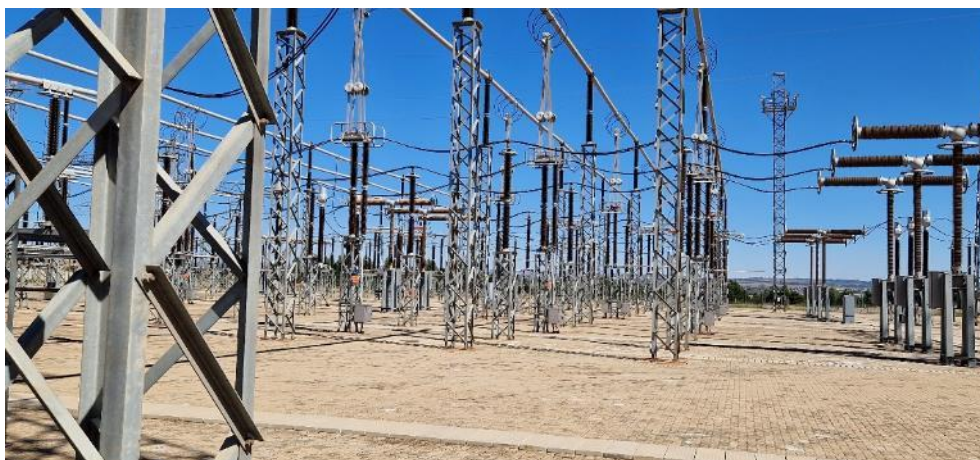
Figure 9-74: 400-kV-switchgear of substation Thuso
