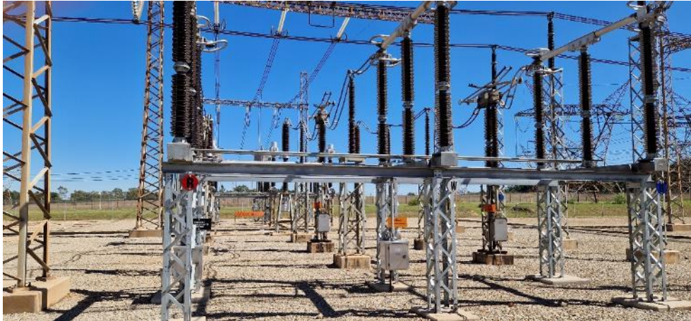
Figure 9-71: Modernized 275 kV switchgear substation Apollo 400/275 kV
