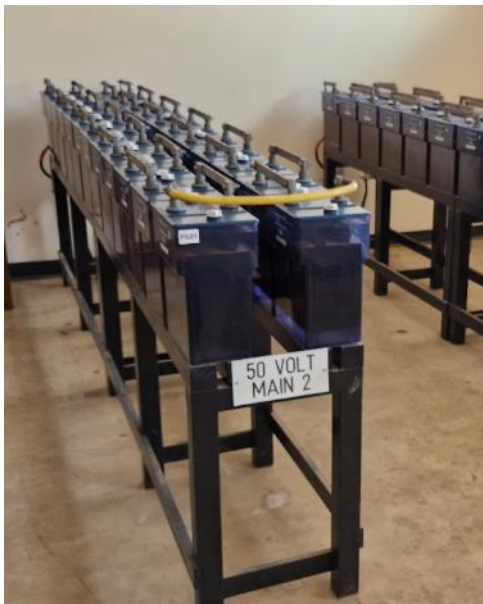
Figure 9-12: Battery systems substation Craighall
