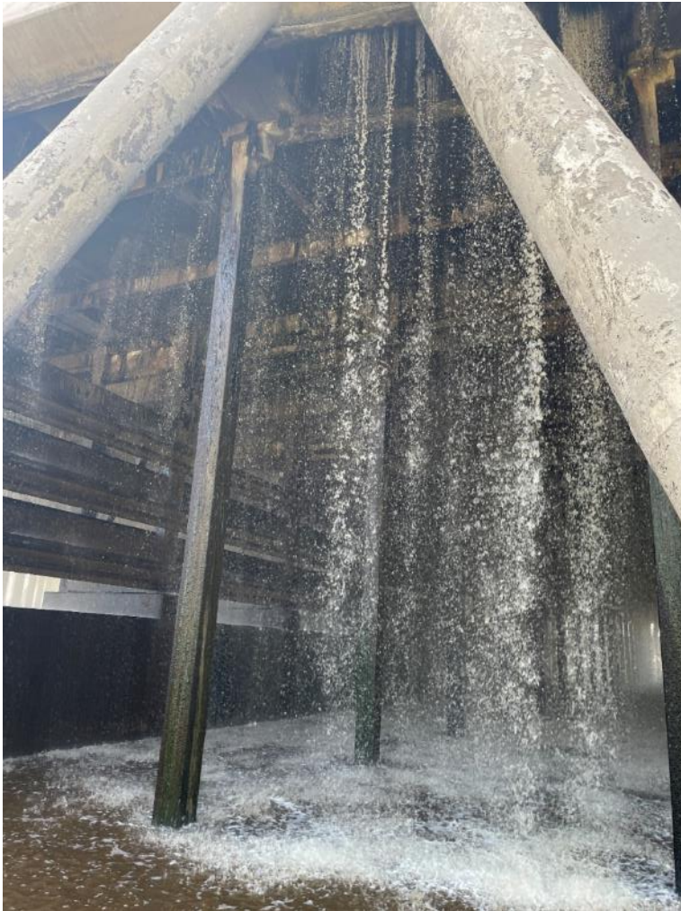
Figure 188: Water distribution and structure of a cooling tower at Tutuka
