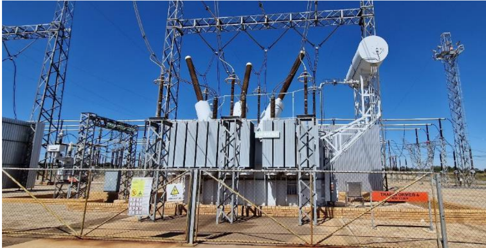
Figure 9-76: Power Transformer 4 of substation Thuso
