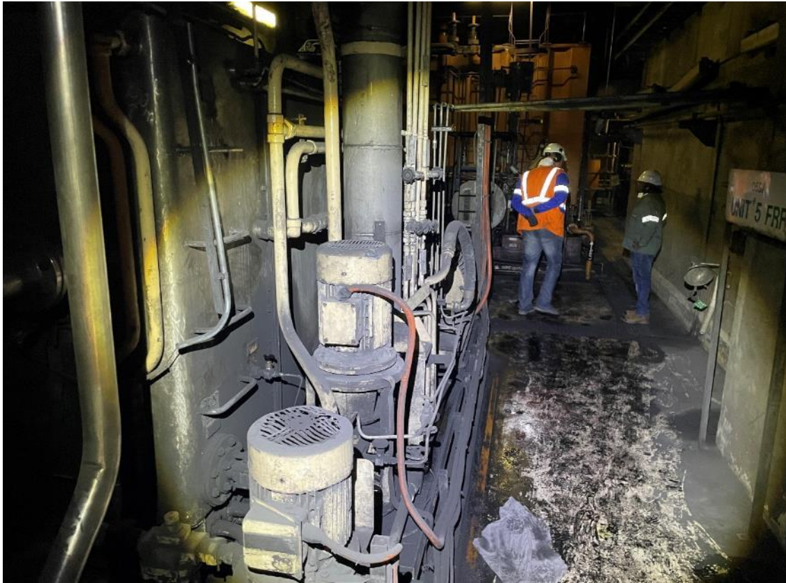
Figure 191: Tutuka's tank room for turbine lube oil – with poor housekeeping
