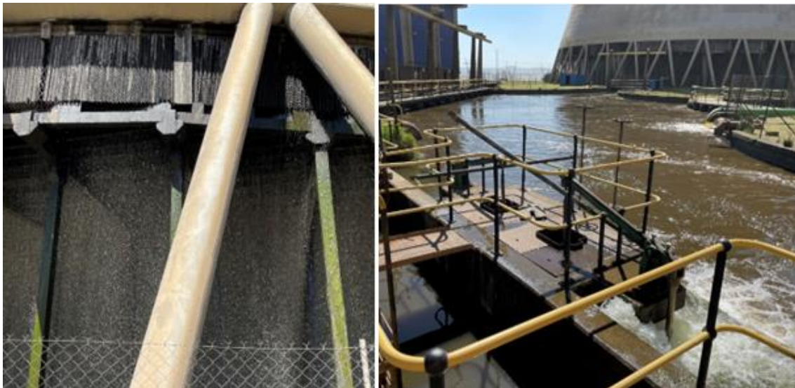
Figure 48: Camden's cooling towers with bio fouling (left) and dirty cooling water (right)
