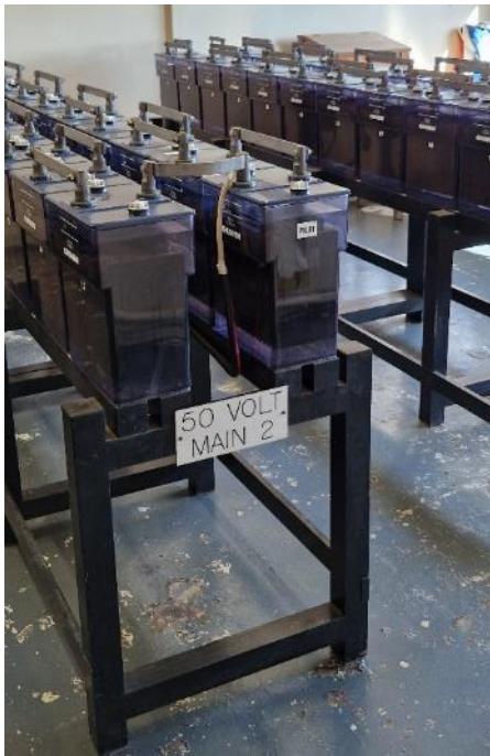
Figure 9-29: 50 V Battery substation Eiger
