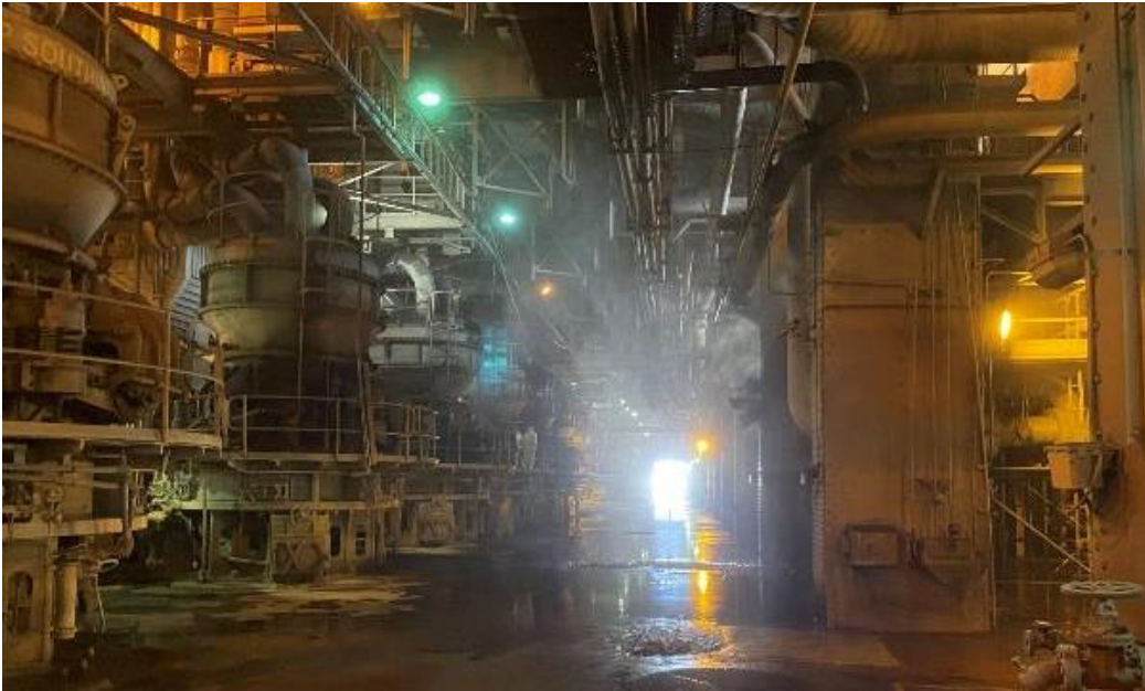
Figure 44: Camden boiler house with steam and water leakages
