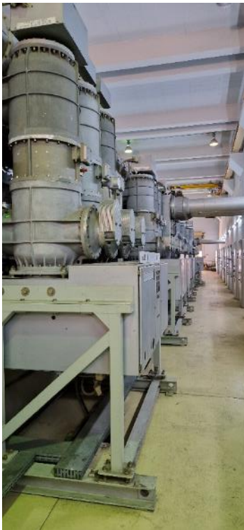
Figure 9-2: 275 kV GIS substation Craighall
