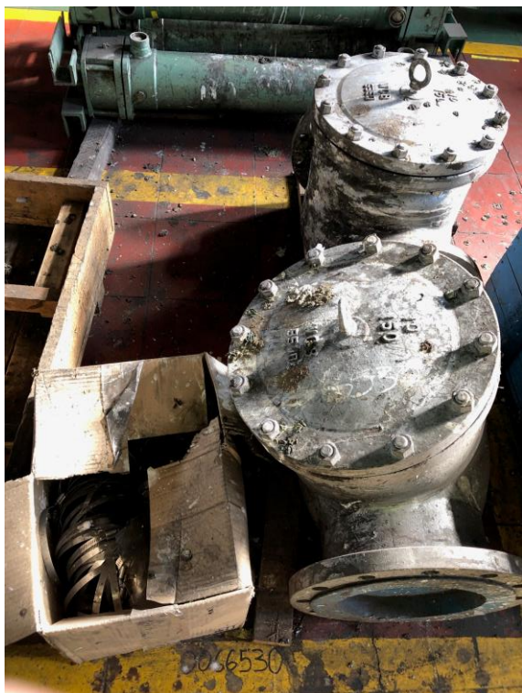
Figure 78: Dirty spare parts at Grootvlei
