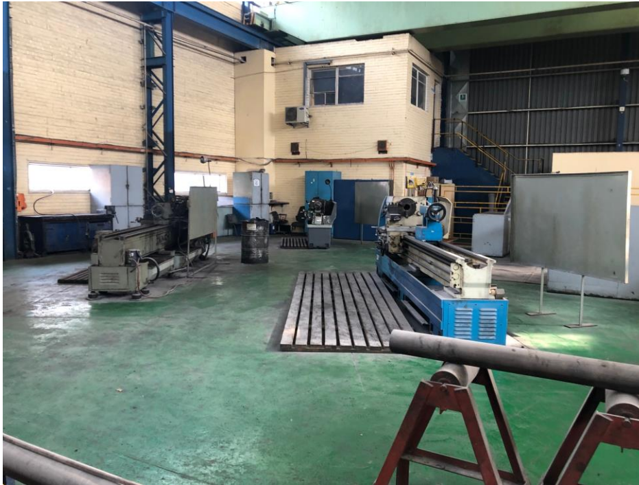
Figure 116: Maintenance workshop at Kriel power plant
