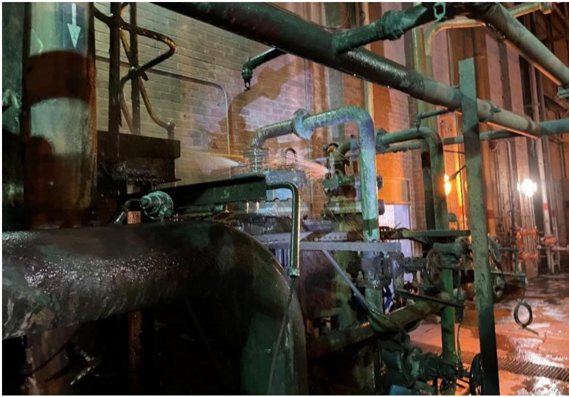
Figure 50: Camden's turbine lube oil cooler with additional external water cooling
