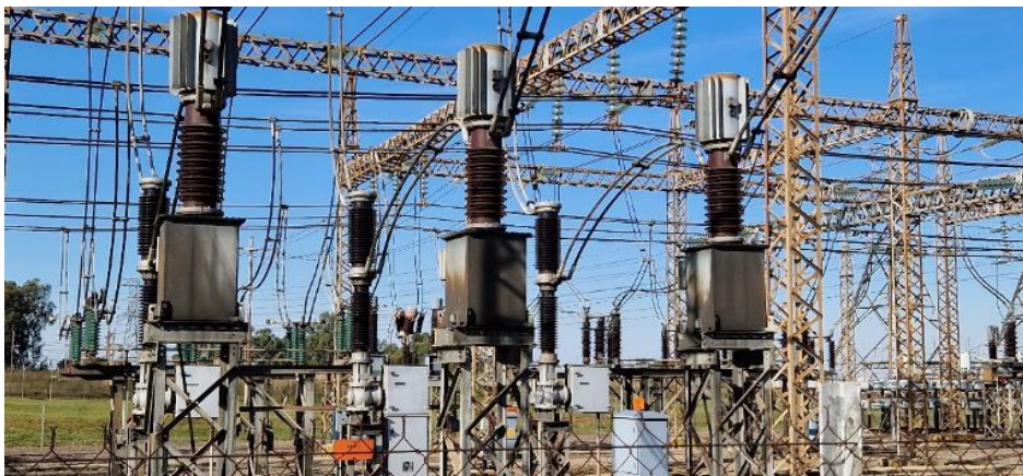
Figure 9-19: 88 kV switchgear substation Eiger
