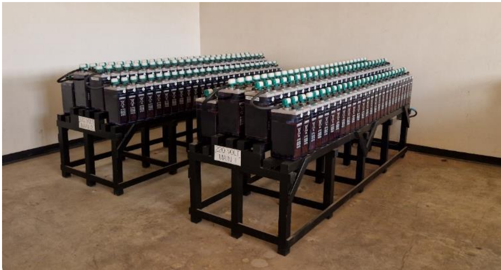
Figure 230: 220 V Battery substation Minerva
