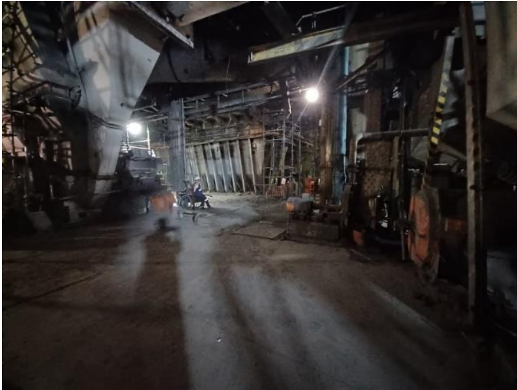
Figure 85: Hendrina boiler at 0 m level
