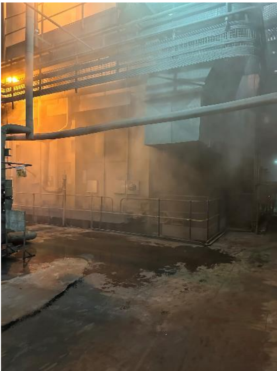
Figure 108: Water and steam leakages in Kriel's boiler house
