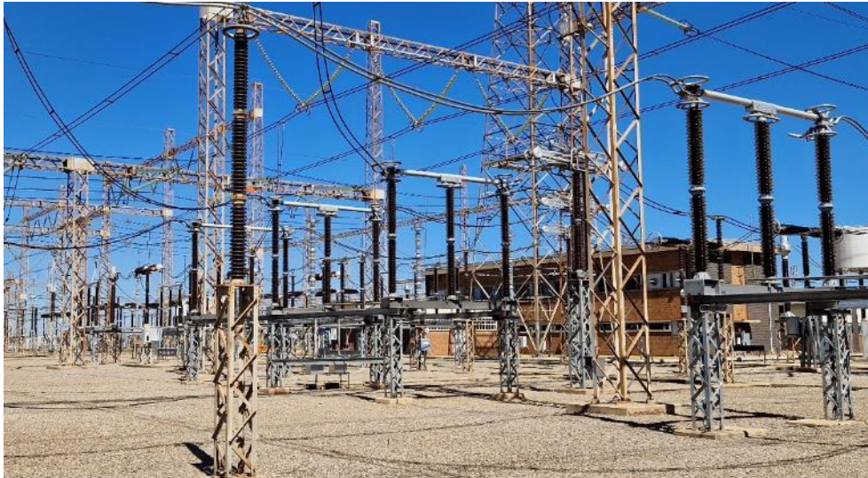
Figure 9-55: Modernized 400 kV switchgear substation Apollo 400/275 kV
