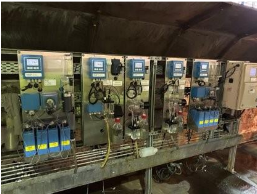
Figure 37: Silica and conductivity measurement in Arnot's make-up water
