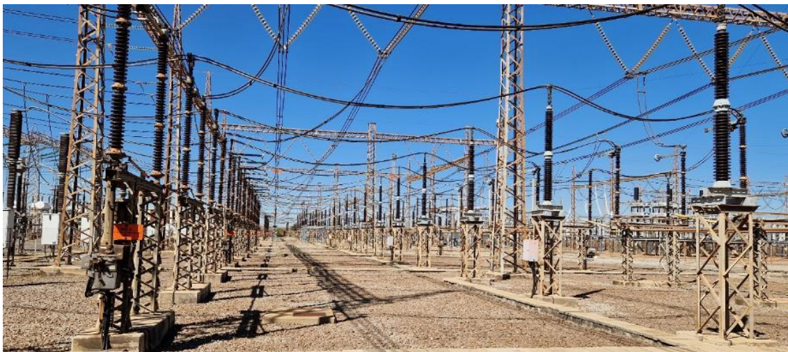
Figure 9-39: 275 kV switchgear Apollo Converter station 530 kV DC/275 kV AC
