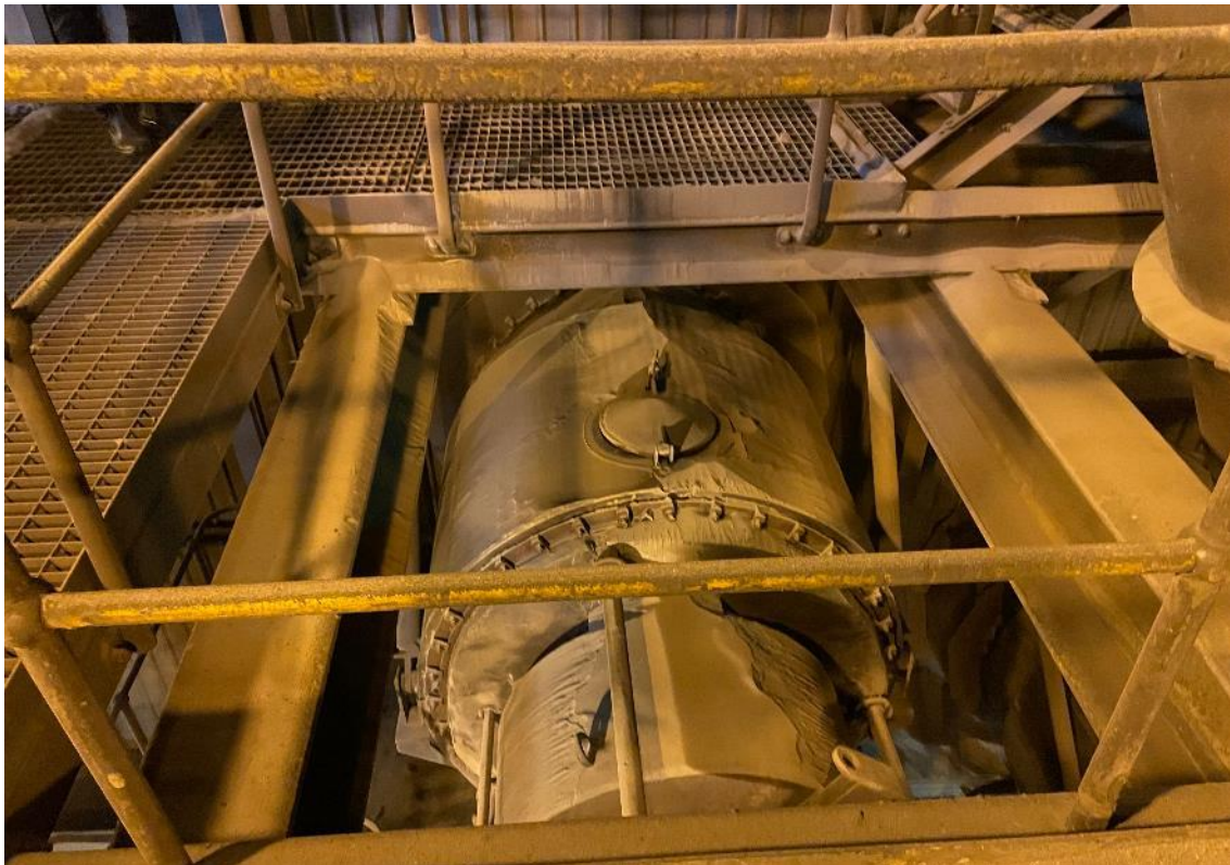
Figure 142: Majuba boilers with a lot of dust due to bad housekeeping
