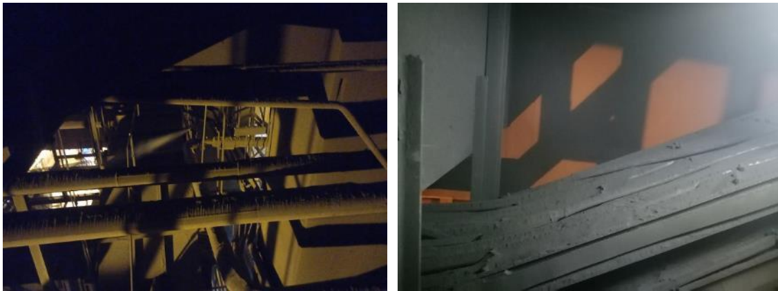
Figure 165: Coal dust on pipes and cable trays at Matla's boiler house
