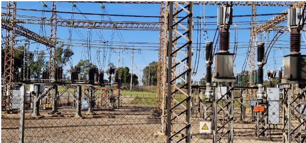
Figure 9-35: 88 kV switchgear substation Eiger
