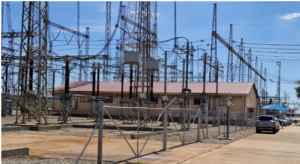
Figure 224: Operation building substation Minerva
