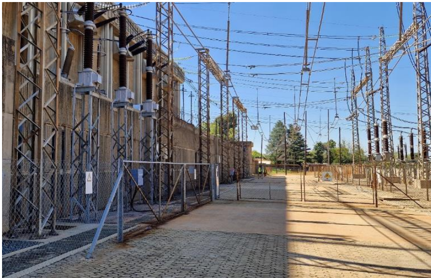
Figure 9-14: Street and fences substation Craighall
