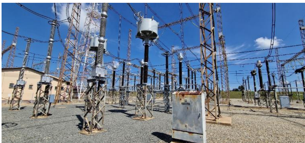
Figure 220: 400 kV switchgear substation Minerva
