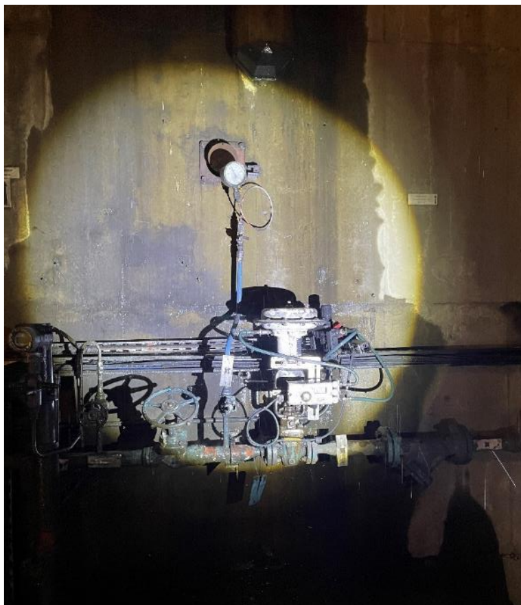
Figure 187: Water/oil leaking on instrumentation and electrical equipment at Tutuka
