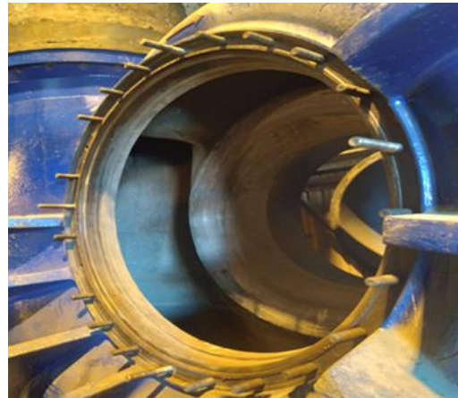
Figure 121: Pump liner failure at Kusile
