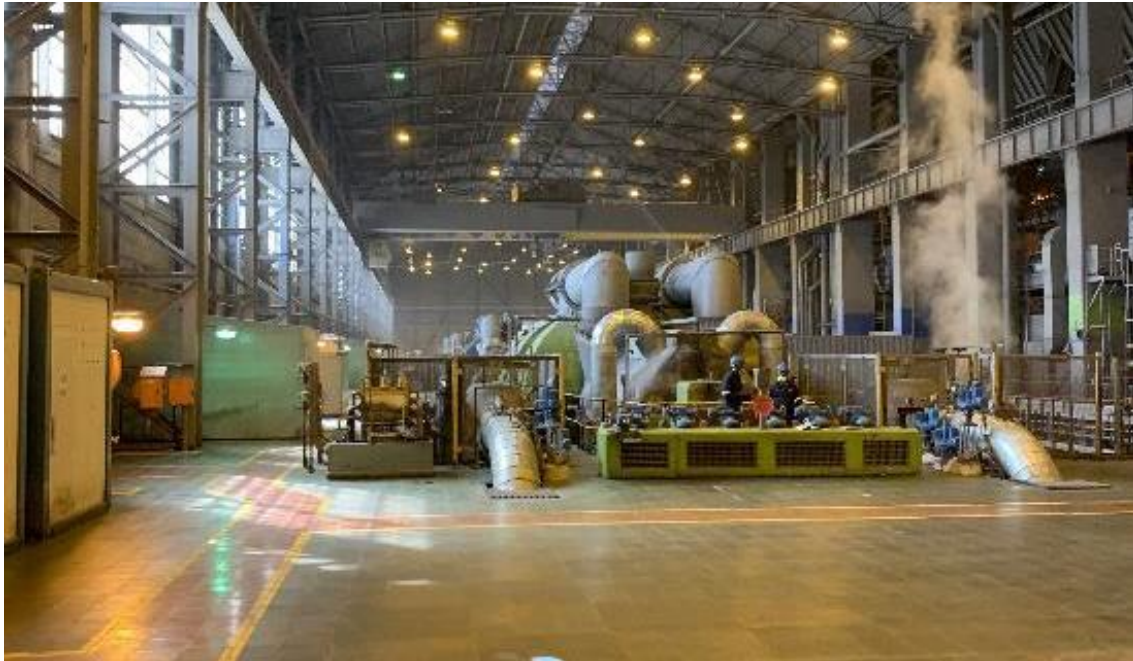
Figure 49: Turbine hall at Camden power plant
