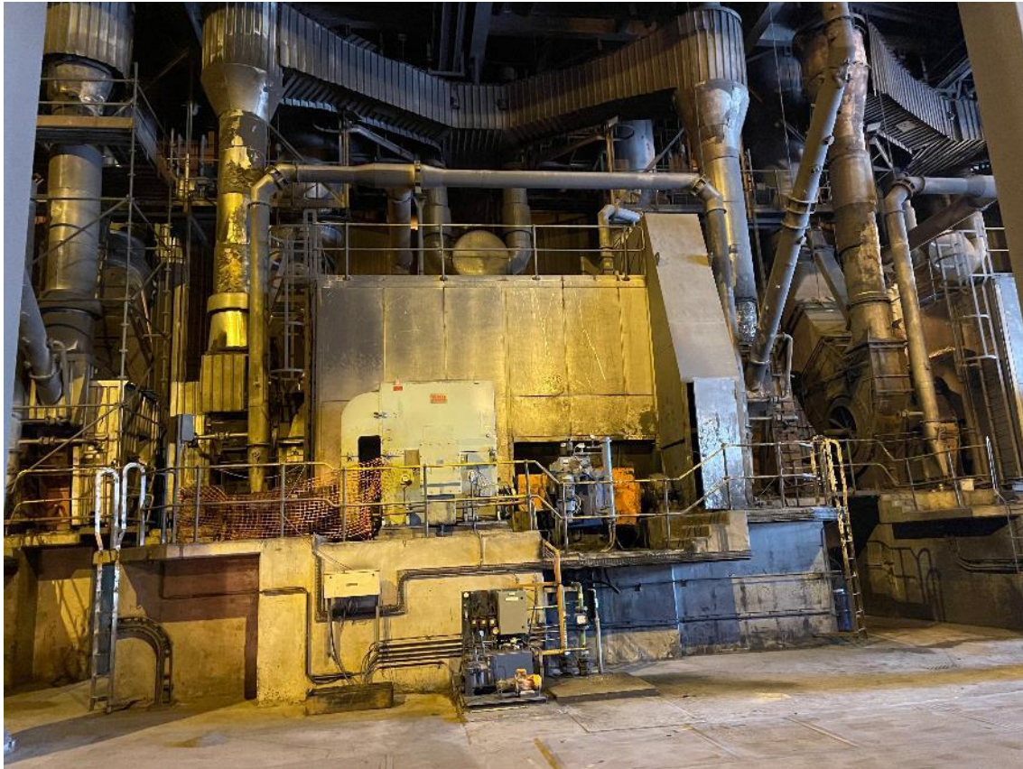
Figure 145: Coal mill at Majuba Unit 1 with patchy canals and overall bad condition
