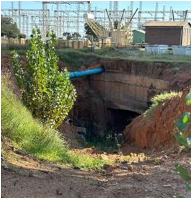
Figure 36: Sinkhole at the Arnot site
