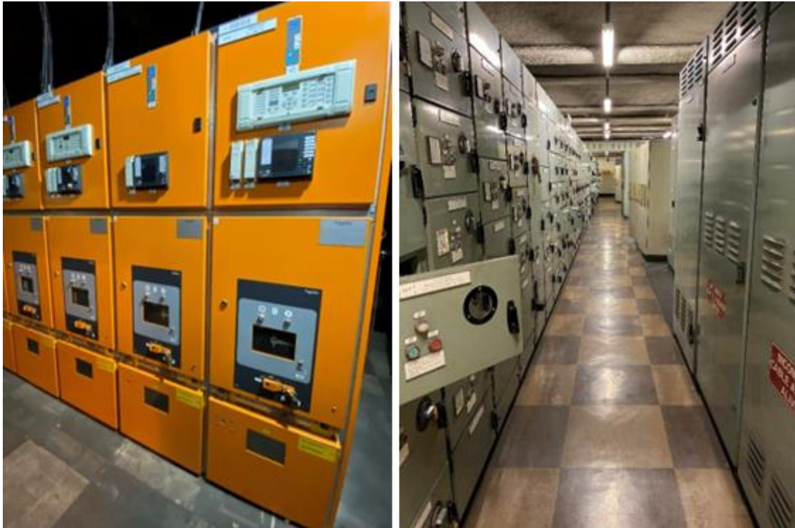
Figure 194: Refurb. MV switchgear (left), non-refurb. switchgear (right) at Tutuka
