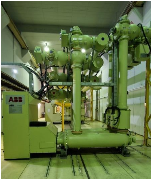
Figure 9-16: 88 kV GIS substation Craighall
