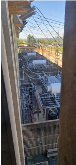
Figure 9-4: Power Transformer substation Craighall
