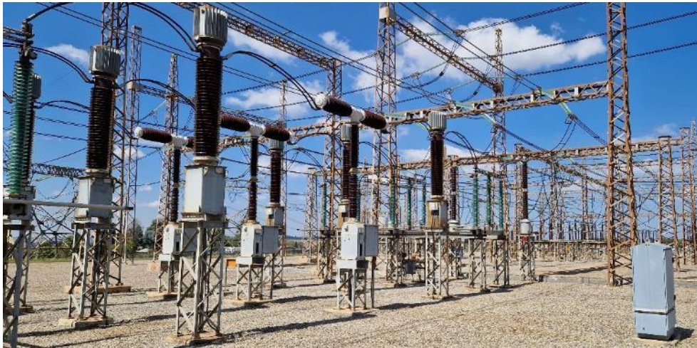
Figure 236: 275 kV switchgear substation Minerva
