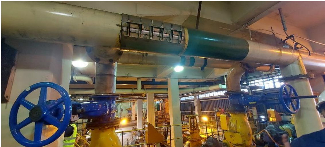
Figure 56: Critical service water line with quick fix installed at Camden power plant
