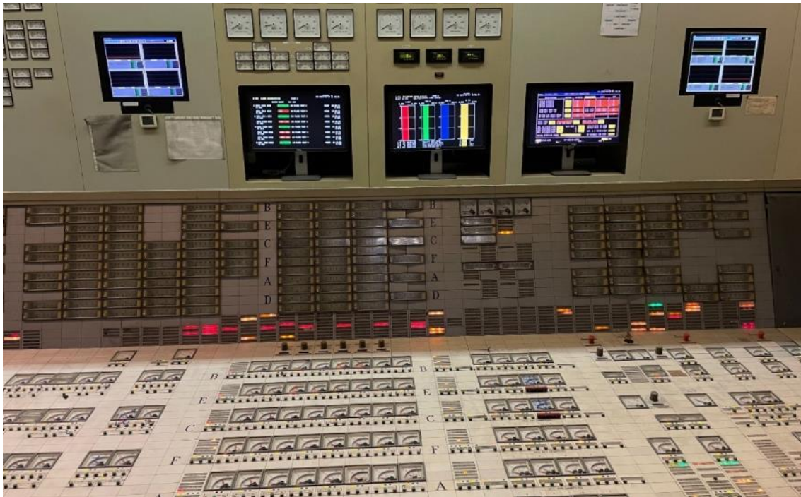
Figure 192: Control room for Units 1 to 3 at Tutuka power plant
