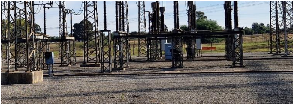
Figure 9-33: Example of Cable duct substation Eiger
