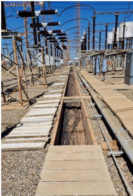
Figure 9-69: Cable duct substation Apollo 400/275 kV
