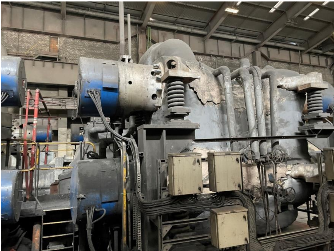
Figure 190: Poorly-cleaned turbine with cracked spray insulation at Tutuka
