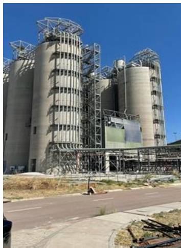
Figure 179: Leakage in silo at Medupi
