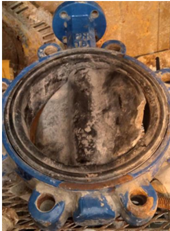
Figure 118: Butterfly valve rubber liner damaged at Kusile
