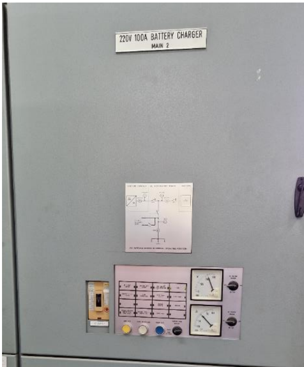
Figure 9-27: AC/DC converter substation Eiger
