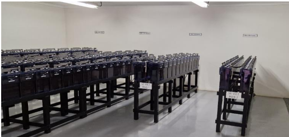
Figure 9-84: Battery room of substation Thuso
