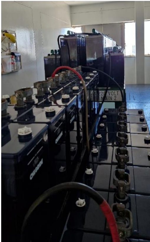
Figure 9-65: Battery system substation Apollo 400/275 kV
