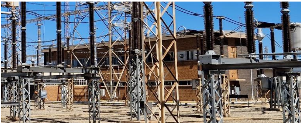
Figure 9-59: Operation Building substation Apollo 400/275 kV
