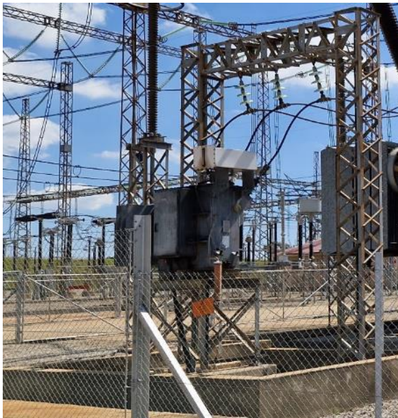
Figure 228: Auxiliary transformer substation Minerva
