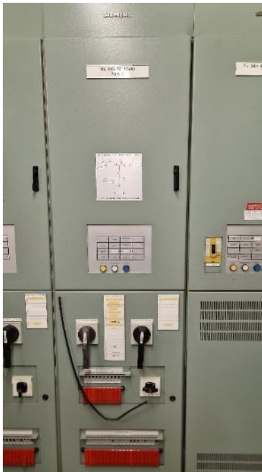
Figure 9-10: AC/DC converter substation Craighall
