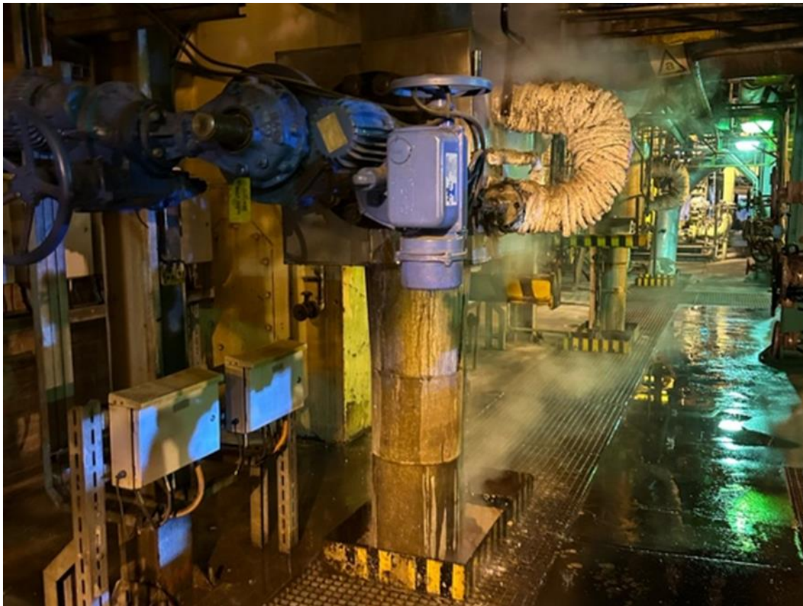
Figure 60: Leakages at Duvha boiler house
