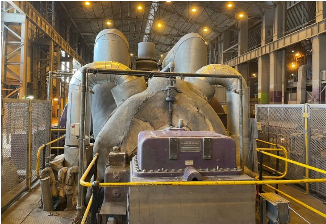
Figure 51: Turbine with cracked spray insulation at Camden power plant
