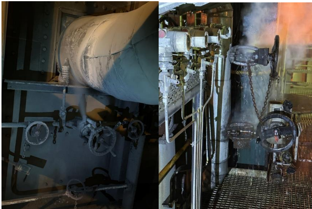
Figure 31: Examples of steam and water leakages in Arnot's boiler house
