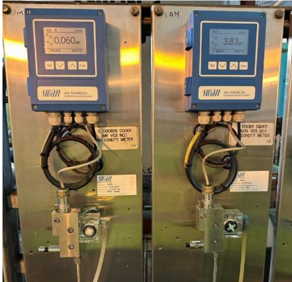
Figure 35: Instrumentation at Arnot's water treatment plant
