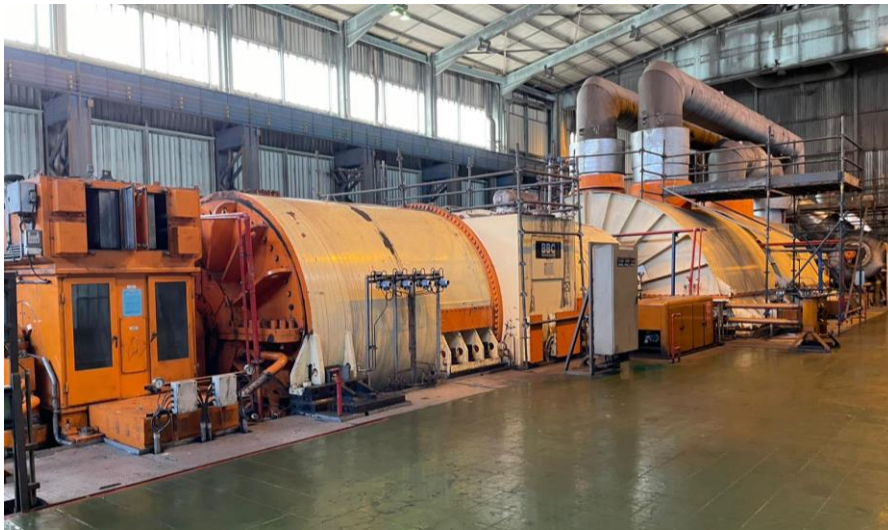
Figure 110: Clean turbine area at Kriell
