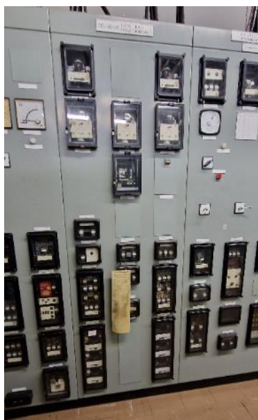
Figure 9-8: Example protection panel substation Craighall
