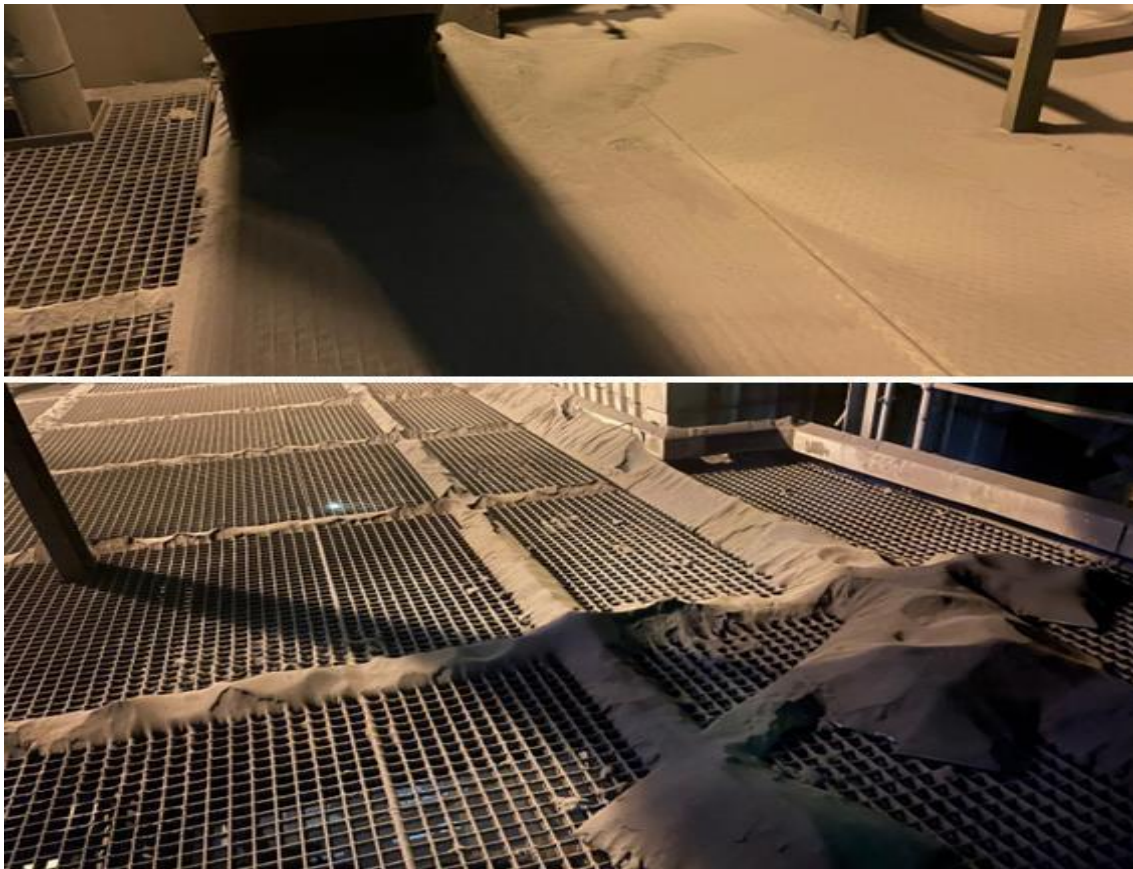
Figure 184: Massive dust pollution at Tutuka's boiler house
