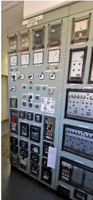
Figure 9-61: Outdated secondary technology substation Apollo 400/275 kV
