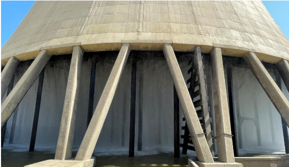
Figure 146: Majuba cooling towers without biofouling and with a proper spray pattern
