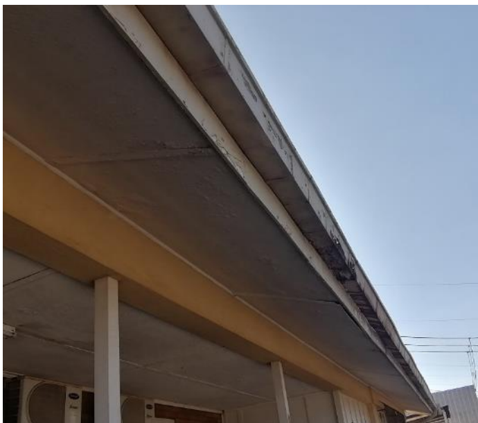
Figure 9-23: Operation Building substation Eiger, small defects of the roof observed
