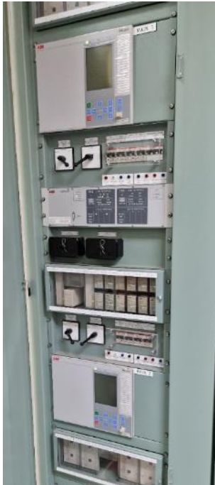
Figure 9-80 Example of a protection cabinet in substation Thuso
