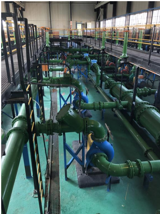
Figure 113: Water treatment plant at Kriel
