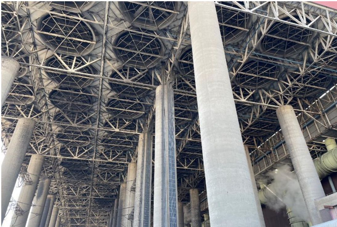
Figure 147: ACC units at Majuba power plant with visible oil residue
