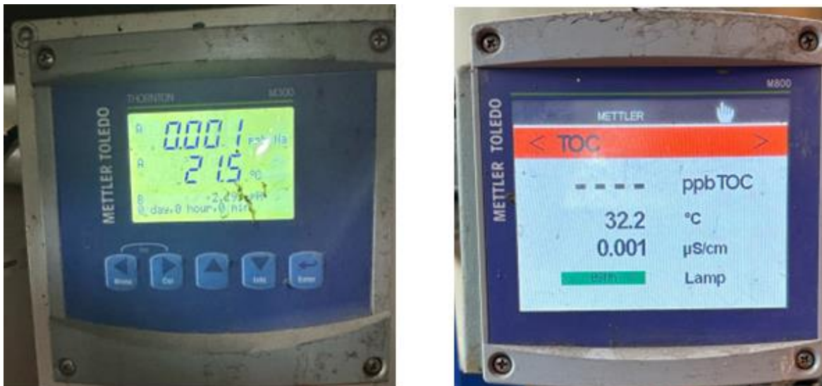
Figure 63: Measurements at the Duvha water treatment plant
