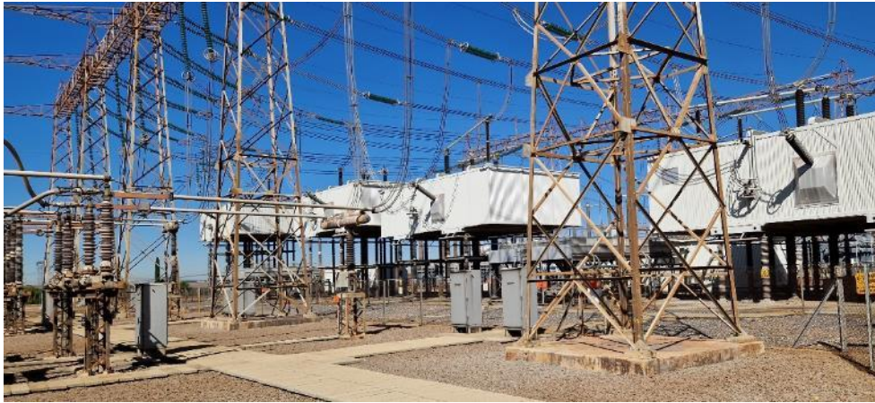
Figure 9-38: Converter Bank Apollo Converter station 530 kV DC/275 kV AC
