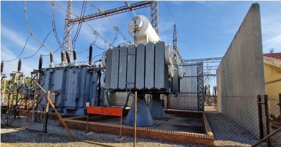
Figure 9-21: Power Transformer 3 substation Eiger
