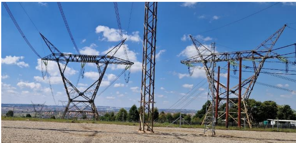
Figure 247: 400 kV OHLs connected to substation Minerva.
