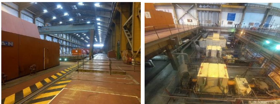
Figure 171: Turbine hall at Matla power plant
