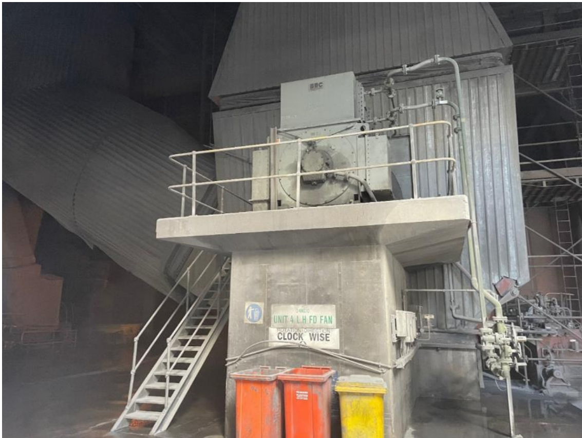
Figure 186: FD fan at Tutuka power plant
