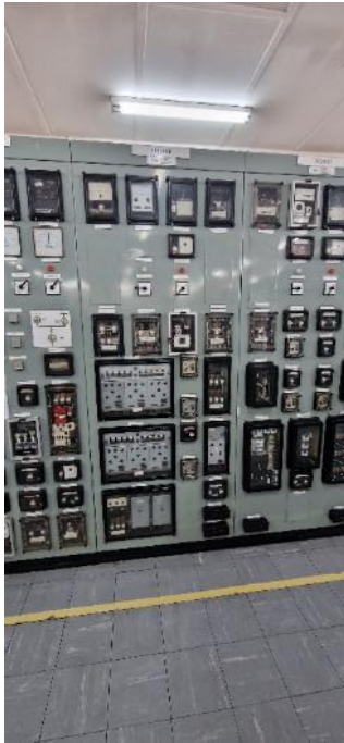
Figure 9-25: Example of control and protection panel substation Eiger
