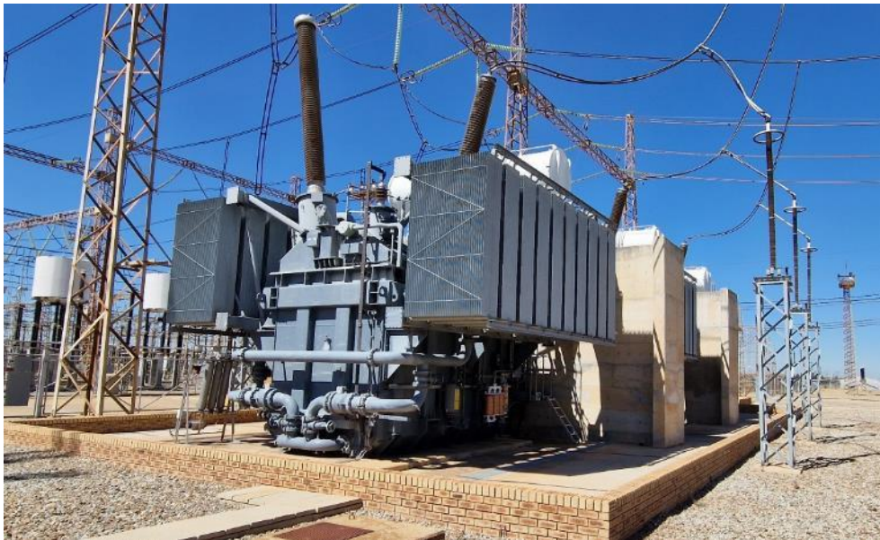
Figure 9-57 Power Transformer pole substation Apollo 400/275 kV
