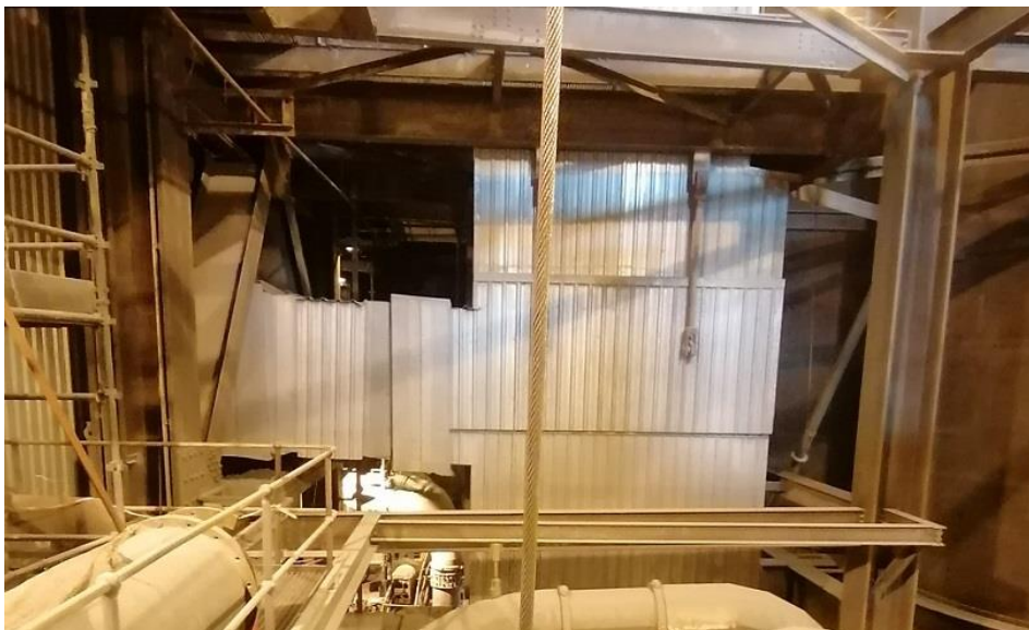
Figure 96: Kendal Unit 4 – same PAH duct not covered in ash and dust (April 2023)
