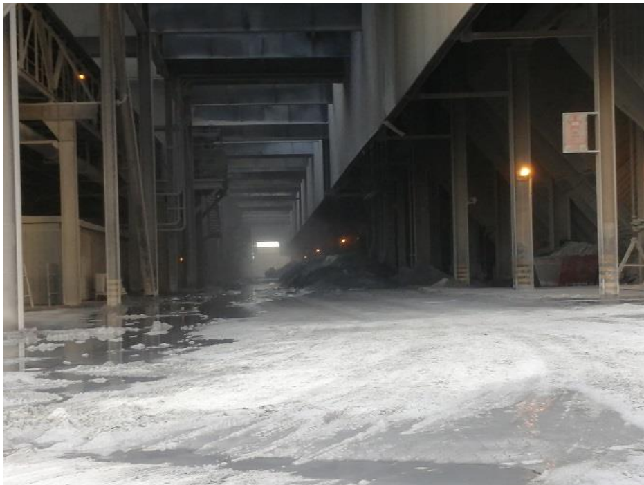
Figure 97: Back of Kendal's boiler at ash handling plant Ash everywhere with water covering the floor. Dust in the air visible: May 2022 26
