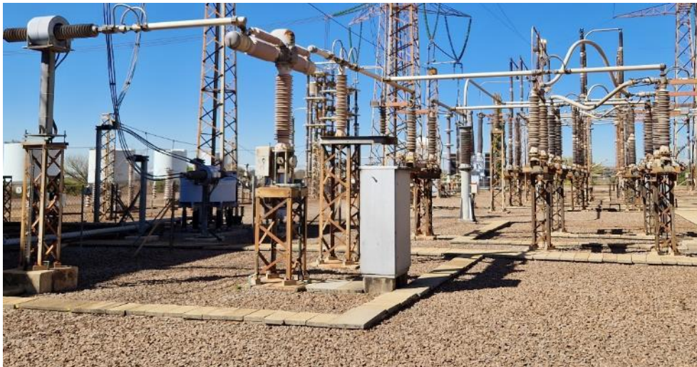
Figure 9-50: Cable ducts Apollo Converter Station 530 kV DC/275 kV AC
