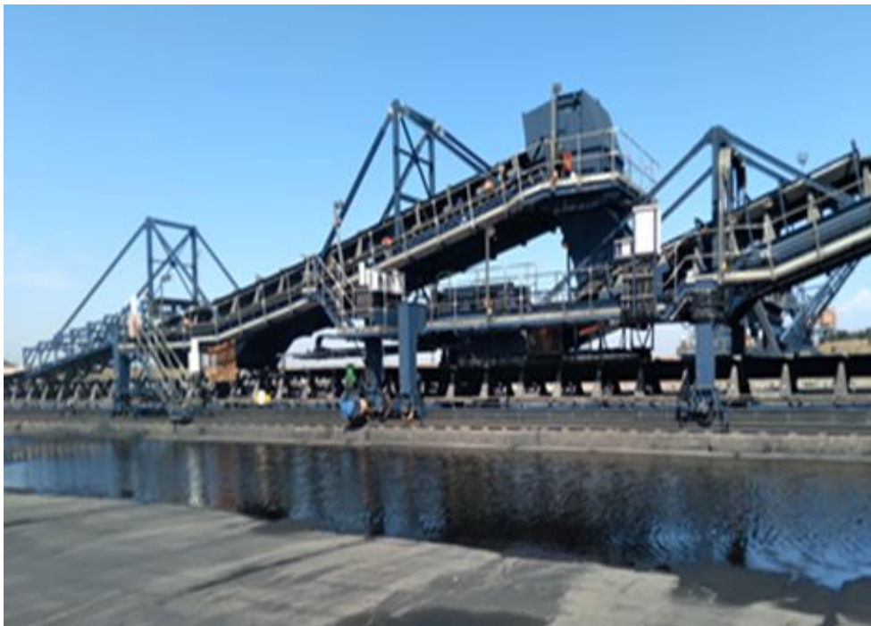
Figure 125: Water logging in Kusile's coal handling plant
