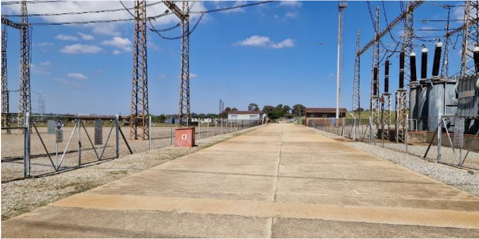
Figure 232: Transportation street and fences substation Minerva
