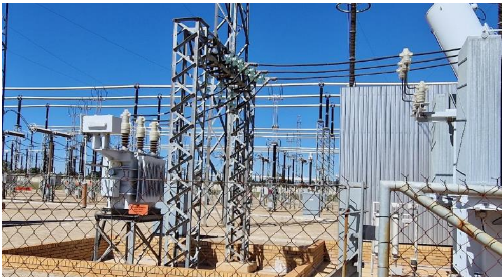
Figure 9-82: Auxiliary transformer as example of one component of the AC/DC system
