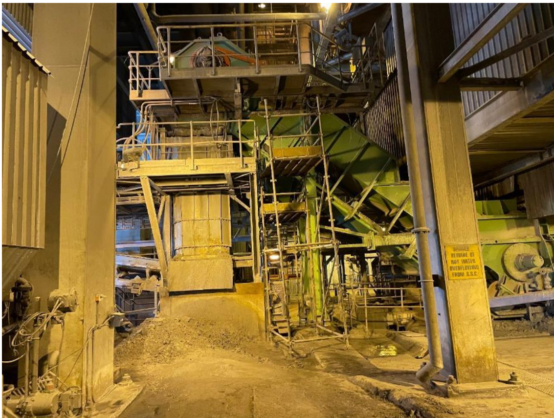
Figure 144: Majuba's ash extraction, emergency disposal – poor housekeeping
