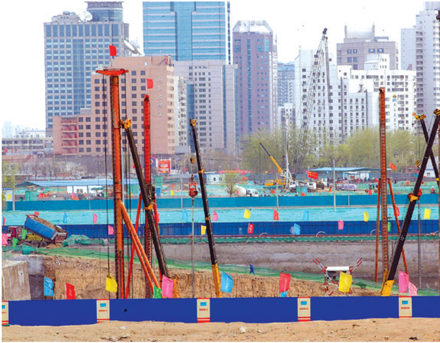
The National Swimming Center, one of the key Olympic sports venues, is due to be completed in 2006.
